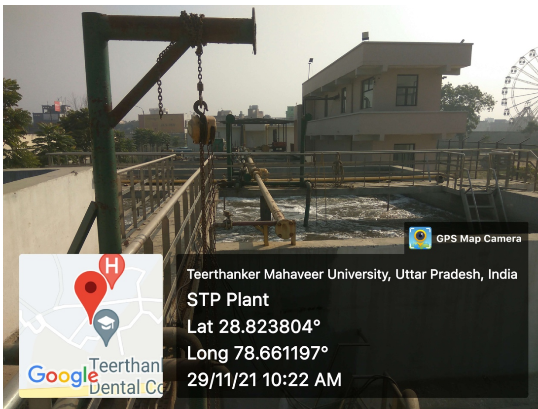
Sewage Treatment Plant
