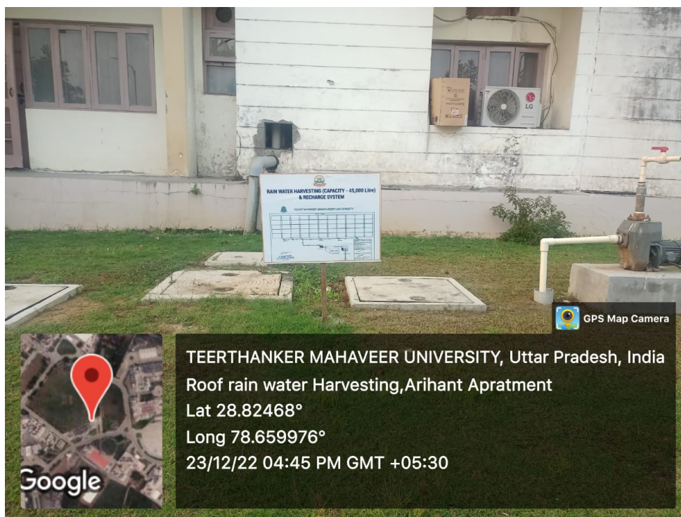
Roof Rain Harvesting
